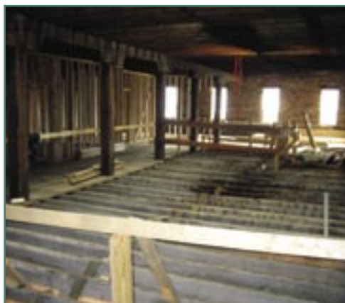
Construction of Phase II of High Street Lofts, located in downtown Petersburg, is now underway.
